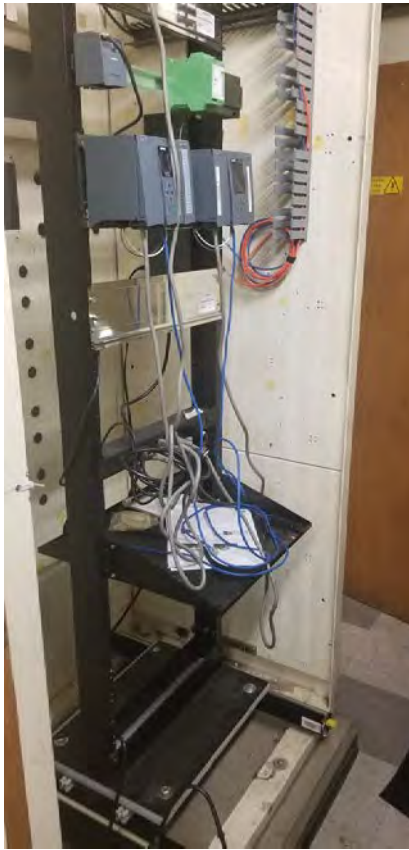
PLC Test Rack (In)
