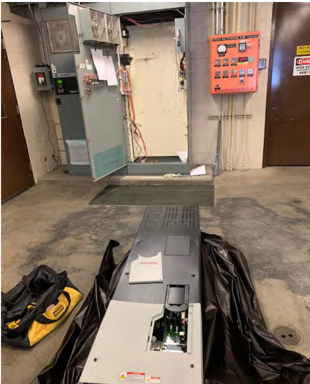
MPPS VFD Replacement
