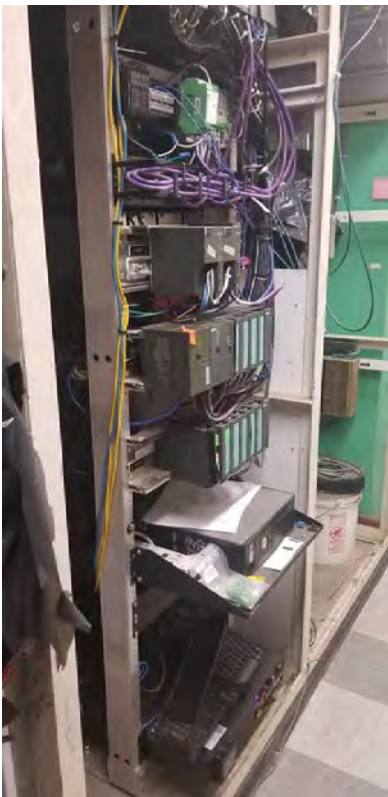
53 PLC Rack to be remounted
