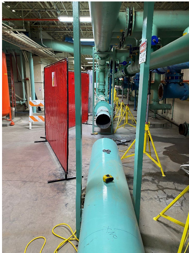
Final Effluent Flow Meter Installation
