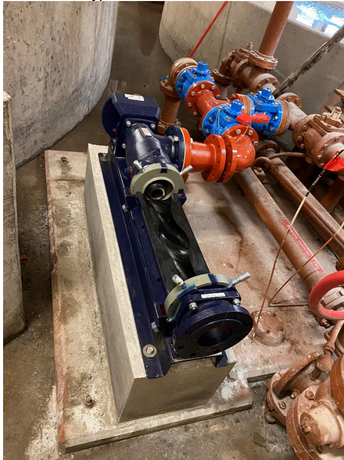
TWAS Pump Installation
