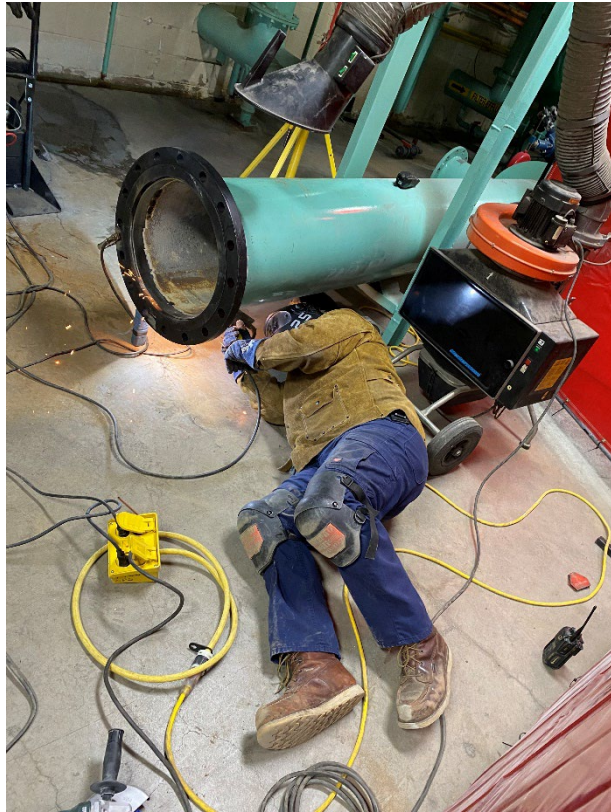
Final Effluent Flow Meter Installation
