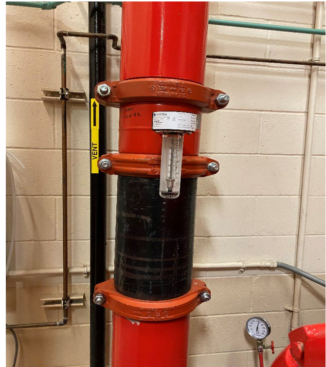
Fire Sprinkler Flow Meter
