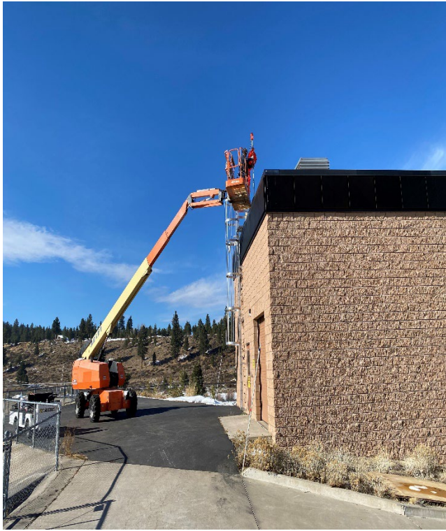
BNR Influent Pump Station Windsock
