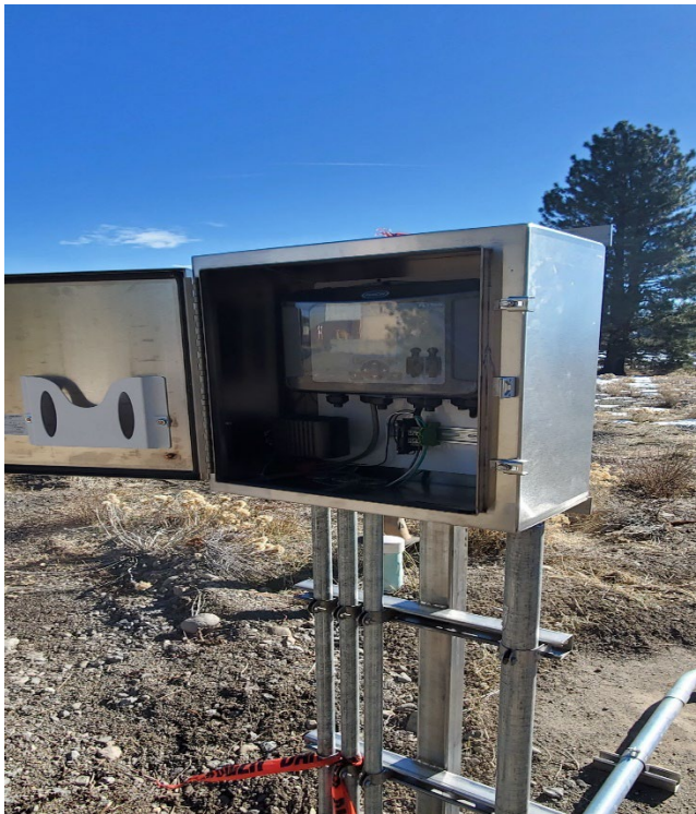
Parallel Line Influent Flodar Panel
