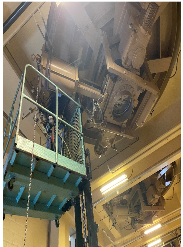
Sludge Load Out Air Cylinder
