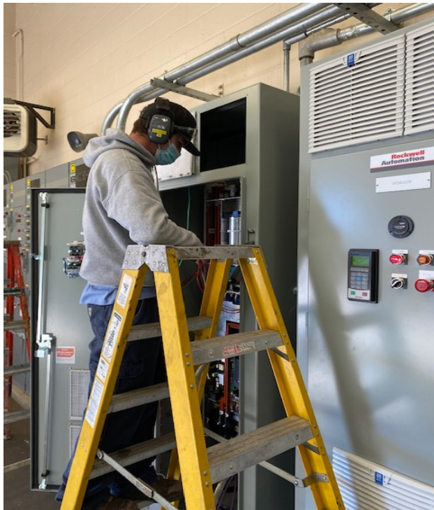
BNR Influent Pump VFD #3
