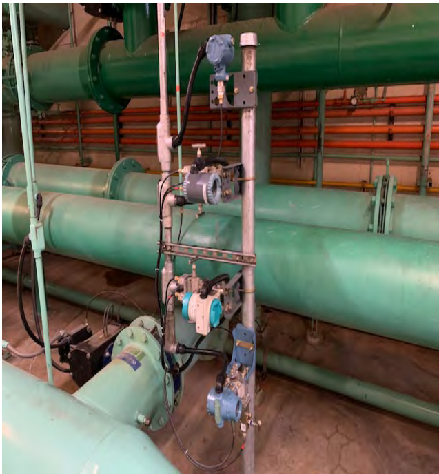
Filter #2 Flow Meter
