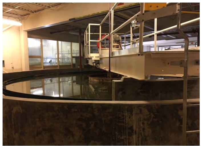
WAS Thickening Clarifier
