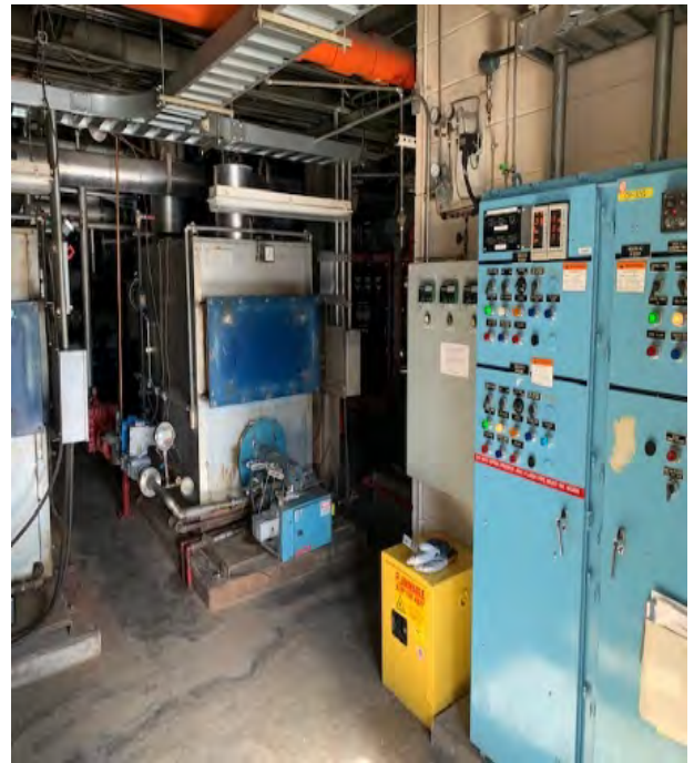
Boiler Control Panel
