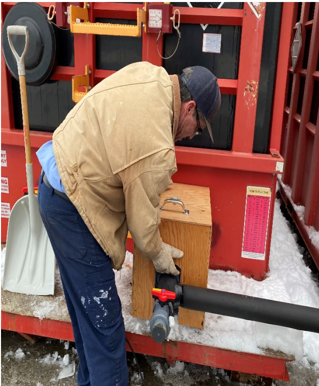
Pipe and Valve Protection
