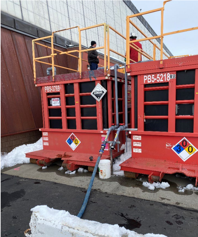
Tank Delivery Area Piping
