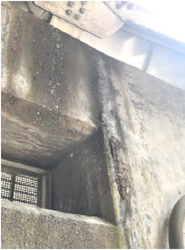
Exposed Rebar in Clarifier 3
