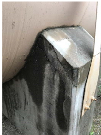
Climo Support Cracks
