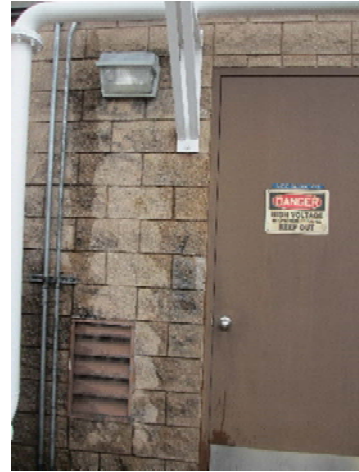
Leaking Wall of MCC Room (13)
