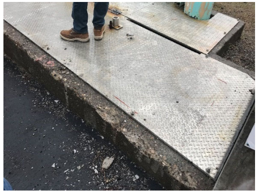
Exposed Concrete Aggregate
