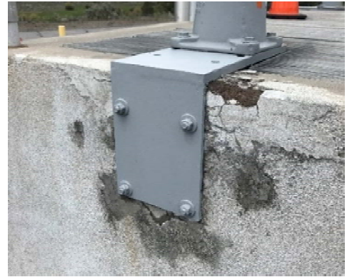
Second Stage Basin Cracking
