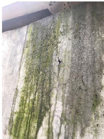
Concrete Cracking and Biological Growth at Roof Connection (Internal)
