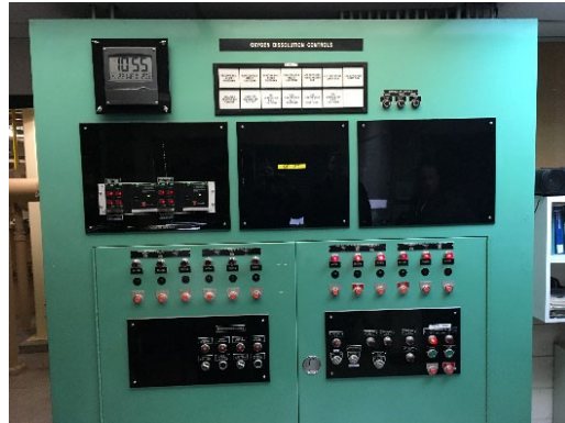
Control Panel 13D
