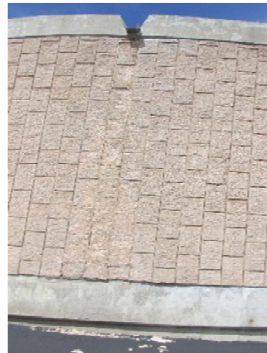
Crumbling Digester No.33 Architectural Finish
