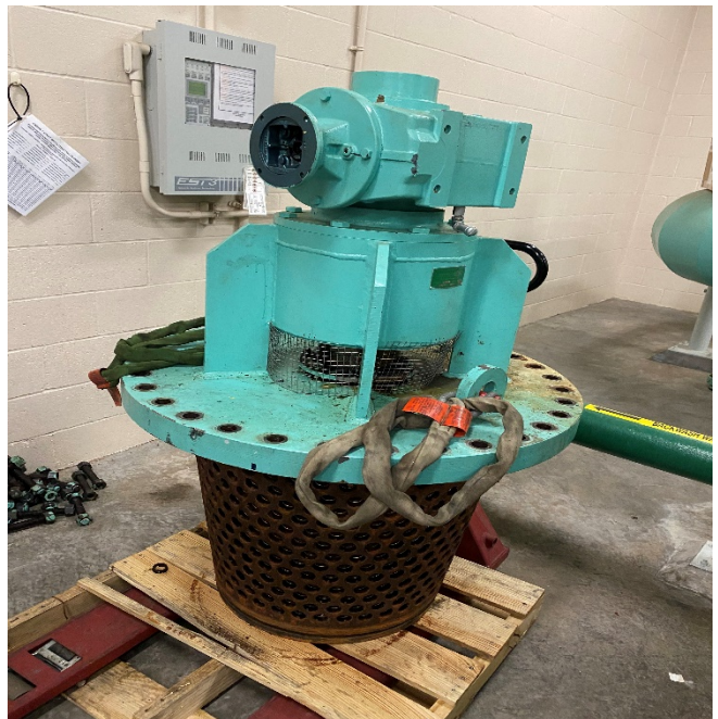
BNR Influent Pump Strainer
