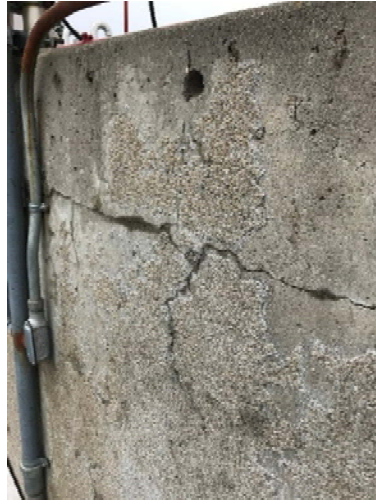
Exterior Wall Surface Delamination
