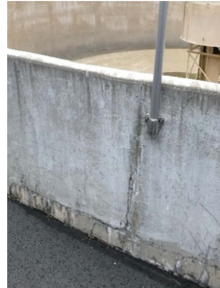
Concrete Cracking of Tank Wall
