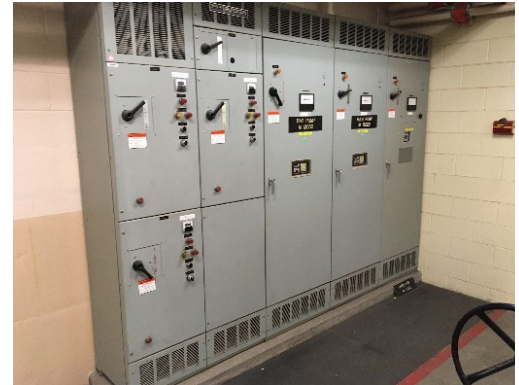
Facility 13 RAS Pump VFDs
