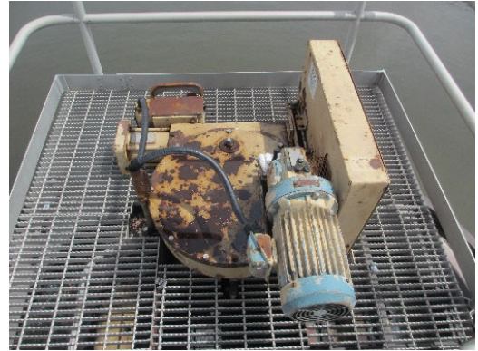
Mechanism Drive Corrosion
