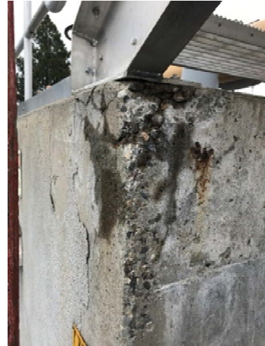
Cracking at Corners
