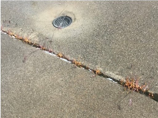
Growth in Construction Joints
