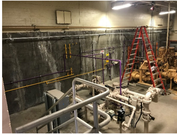
Leaking Wall in Pump Room (53)
