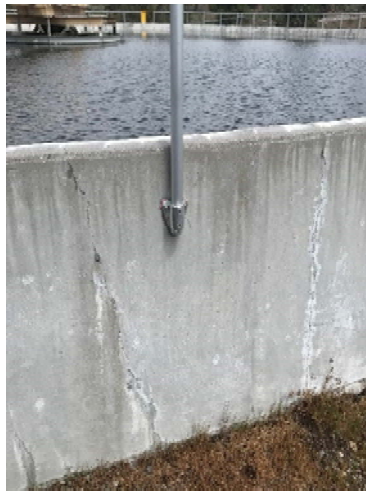
Clarifier 1 Wall Cracks
