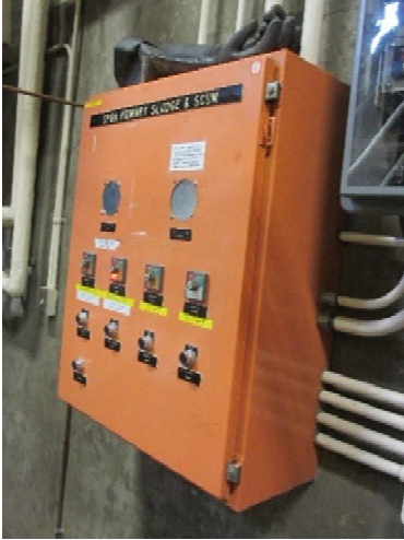
Pump Station 9 Control Panel
