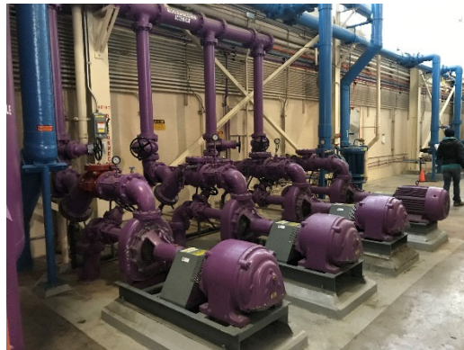
2W Pump Station
