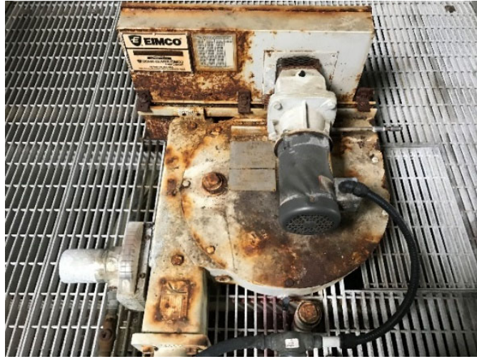
Clarifier No.4 Mechanism Drive
