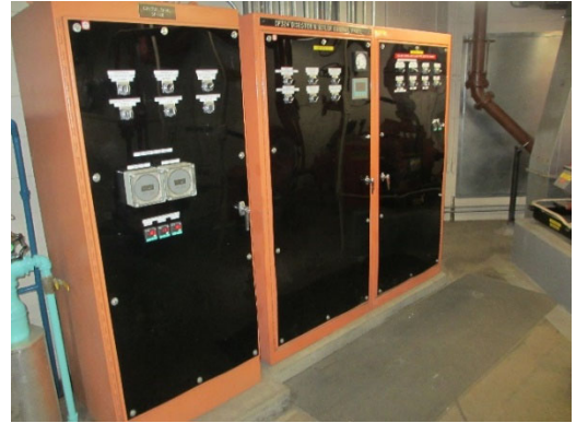
Older Digester and Boiler Control Panels
