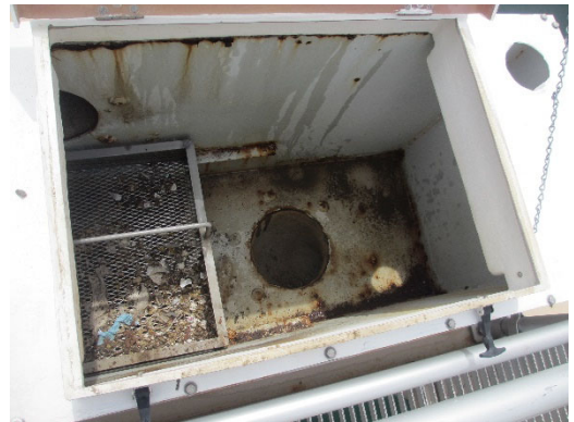
Corrosion Inside Basin 64 Box
