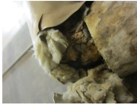
Corroded Pipe Under Insulation
