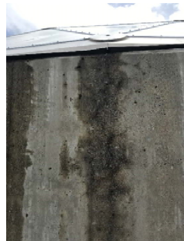
Concrete Cracking and Moisture at Roof Connection (External)
