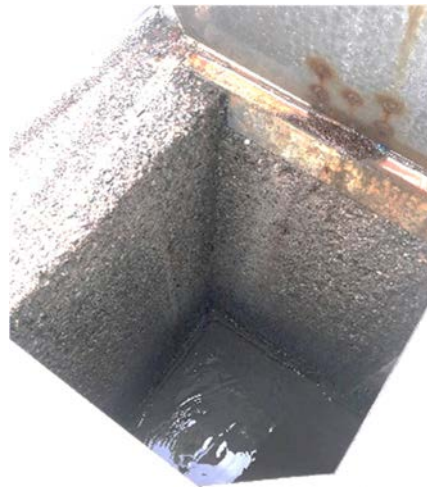
RAS Inlet Corner of Splitter Box
