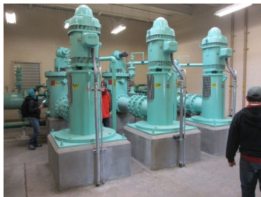
BNR Influent Pumps
