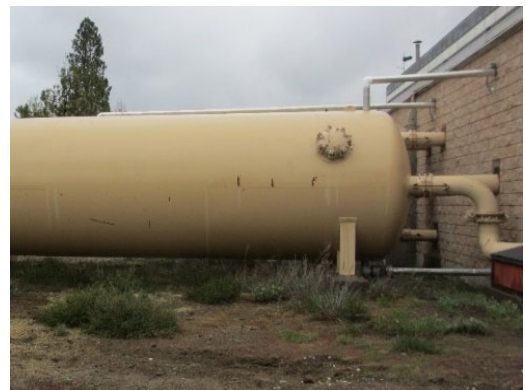
Breakpoint Chlorination Tank
