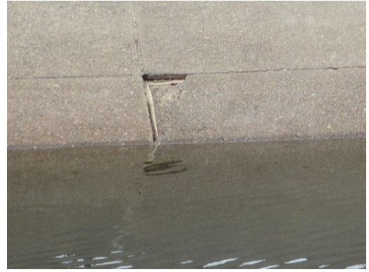
Ballast Pond Joint
