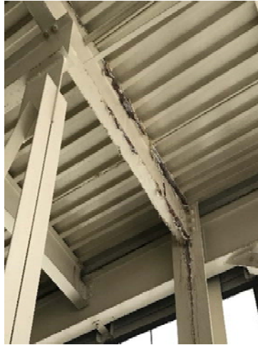
AWT Building Beam Corrosion
