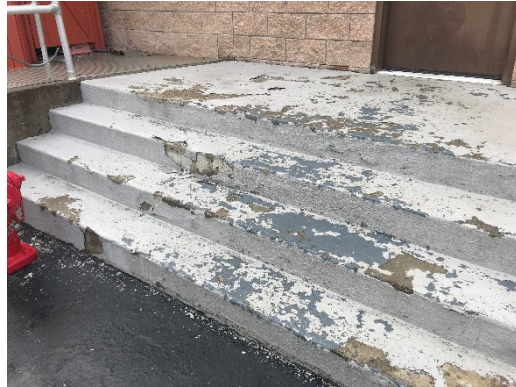
Spalling Concrete on North Stairs
