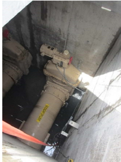
Effluent Valve Vault
