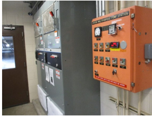
MPPS Cabinet and Control Panel
