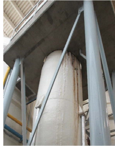
Stripper Duct Damage
