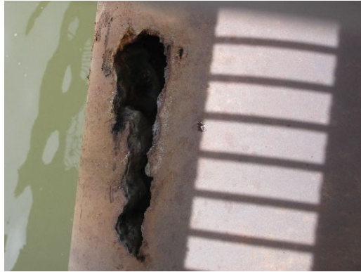
Hole in Elutriant Pipe
