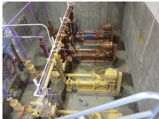
Pump Station 9 Equipment
