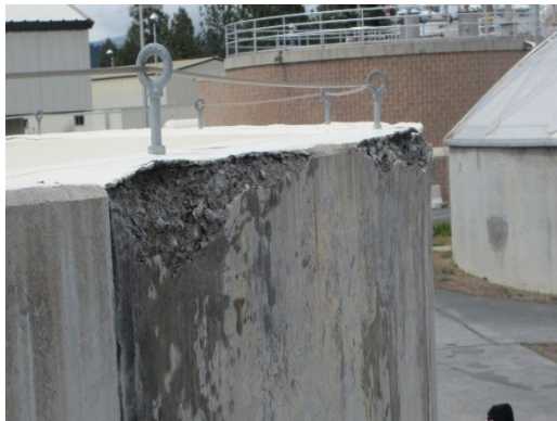
Cracking at Top of Basin 64 Wall
