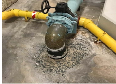
AWT Building Floor Acid Erosion
