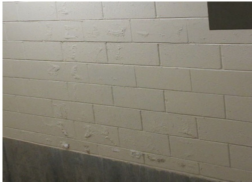
Peeling Paint on CMU Wall
