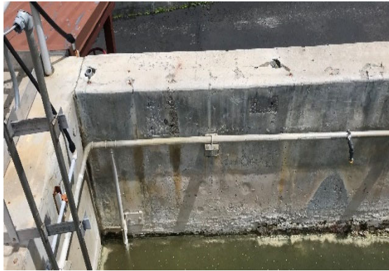
First Stage Basin Concrete Cracking
