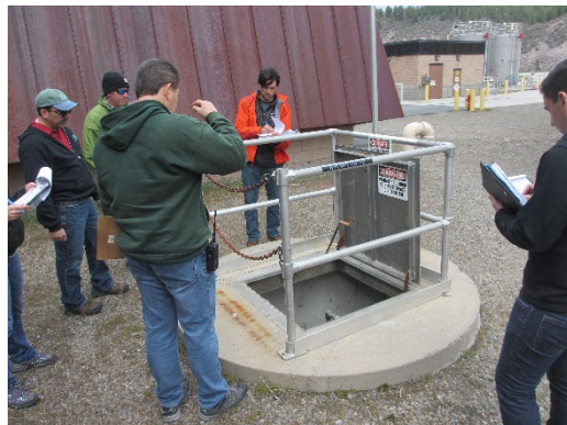
Plant Waste Pump Station
