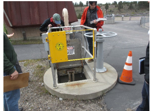
Plant Dewatering Pump Station
