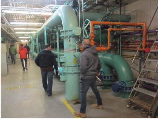
Indoor Filter Piping
