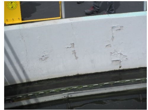
Clarifier 4 Wall Cracks
