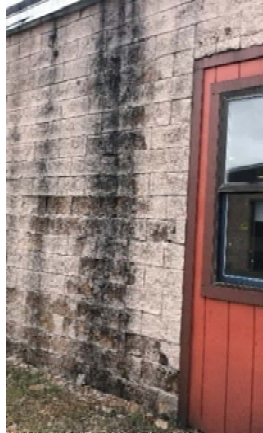
Solids Handling Building CMU Wall Damage
