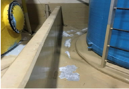
Chemical Containment Coating Failure
