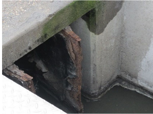
Corroded 1975 Deflector Vane
