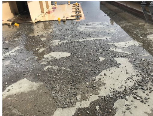
Surface Cracking on Roof Deck
