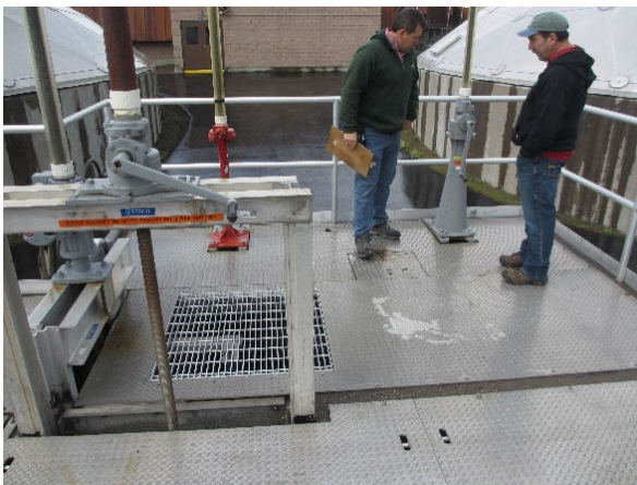
Influent Splitter Box Area
