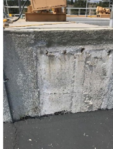
Concrete Wall Damage
