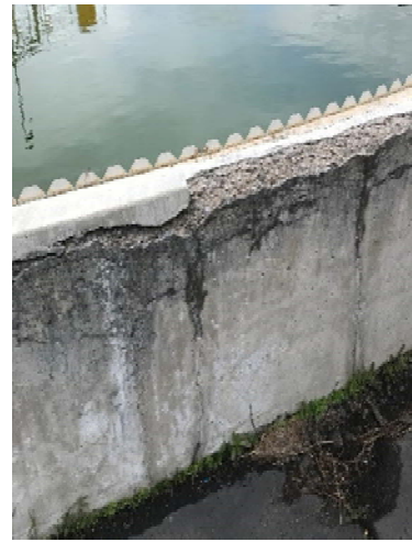
Clarifier 2 Wall Damage
