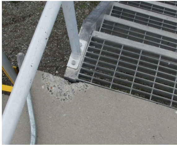
Spalling at Stair Connection
