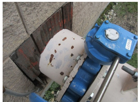
Minor Filter Pipe Corrosion
