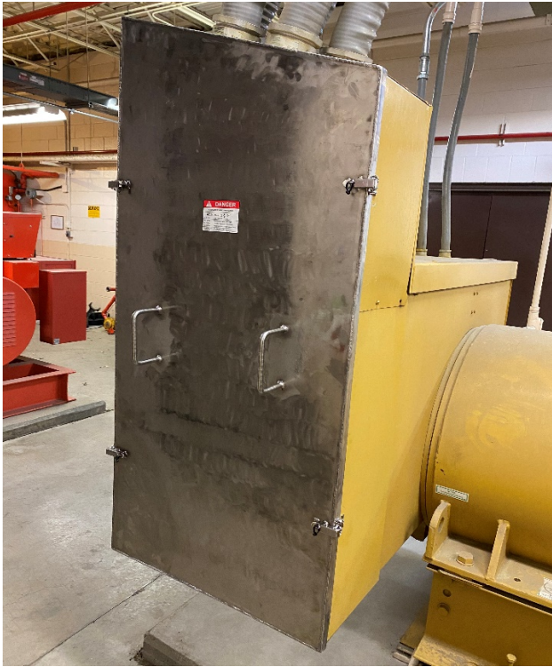
Emergency Generator Panel Door
