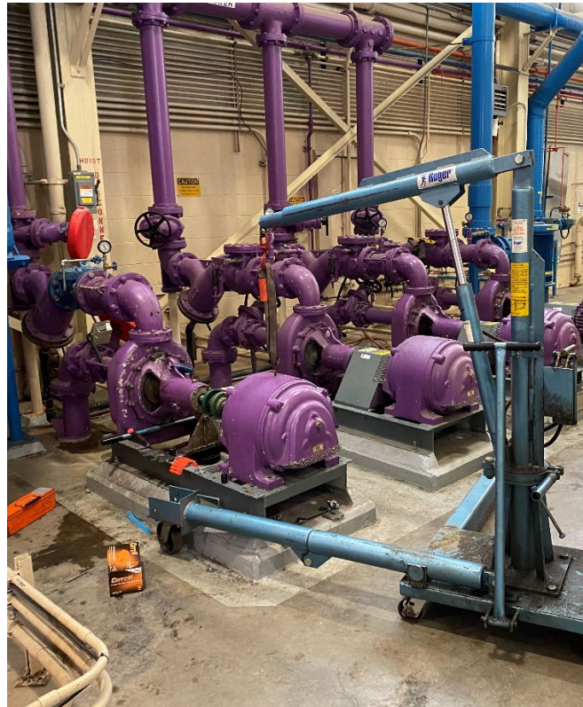
2 Water Pump Installation
