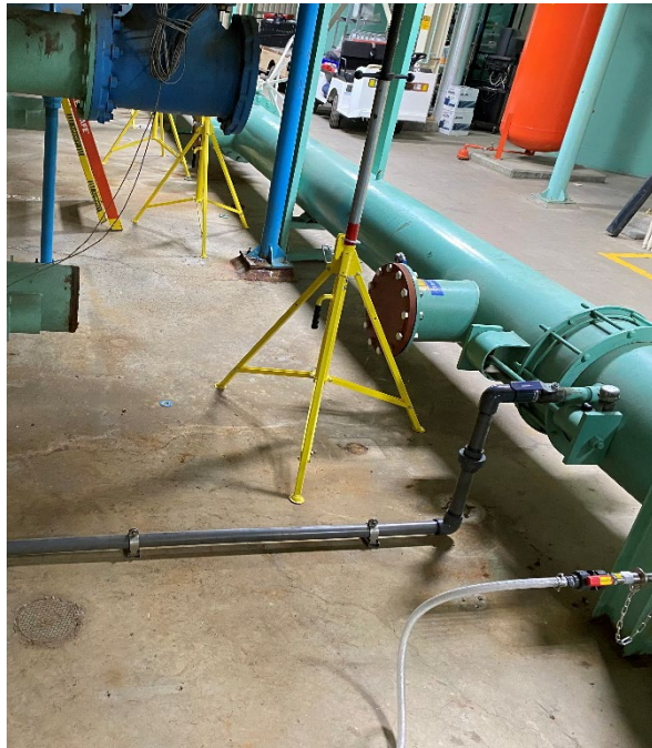
Final Effluent Instrumentation Sample Line
