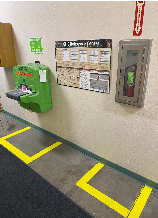
Fire extinguisher and eye wash clearance
