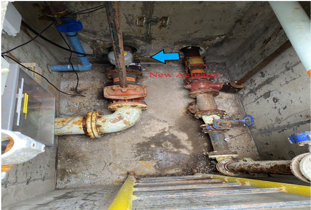
Actuator at 2 Water Pond
