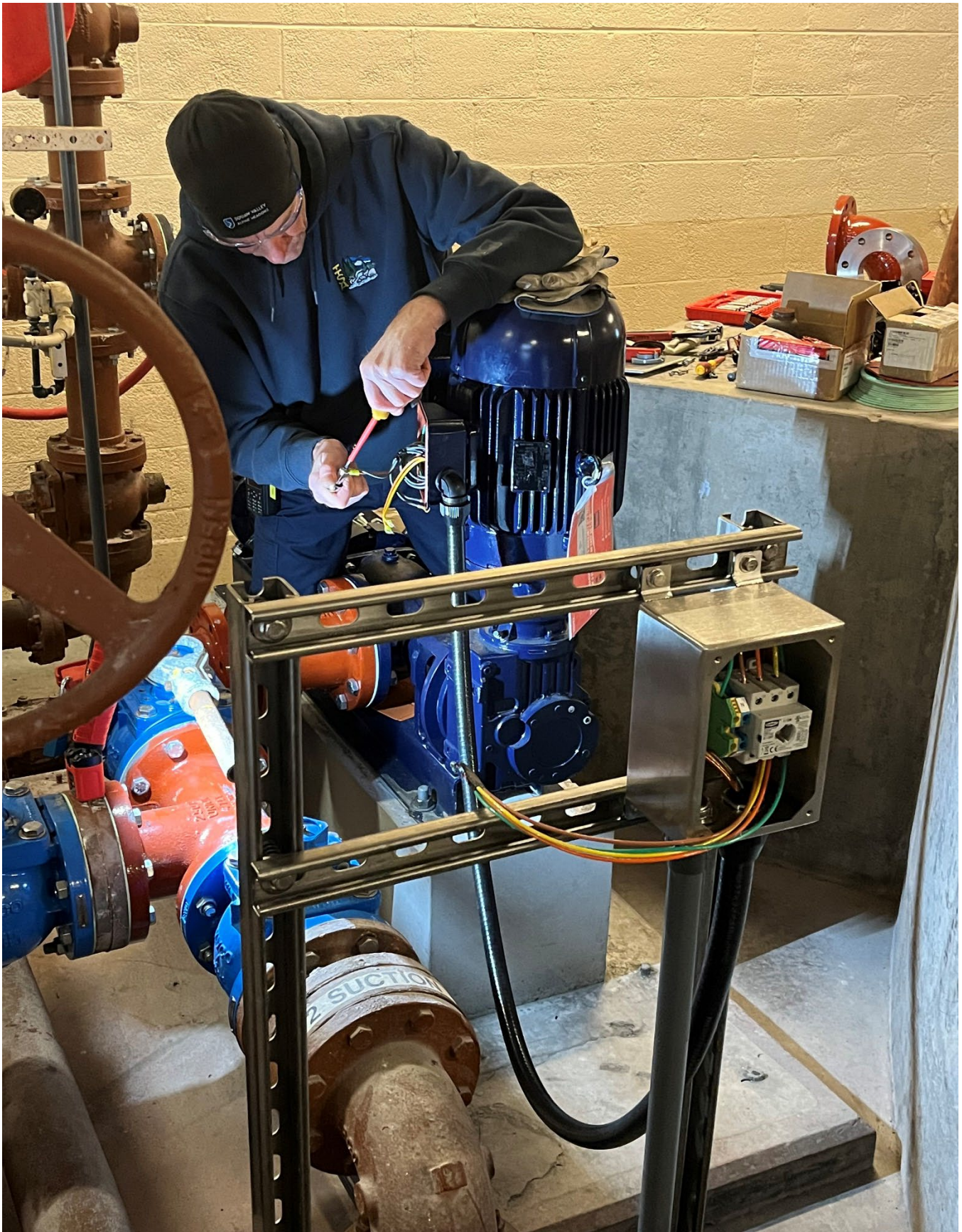
TWAS Pump Installation
