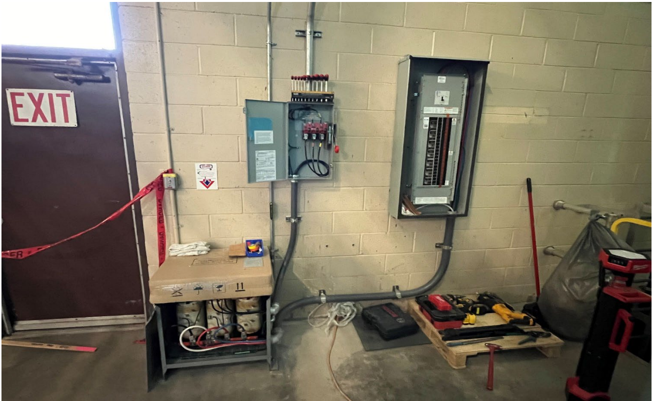
Sodium Hypochlorite Electrical Installation
