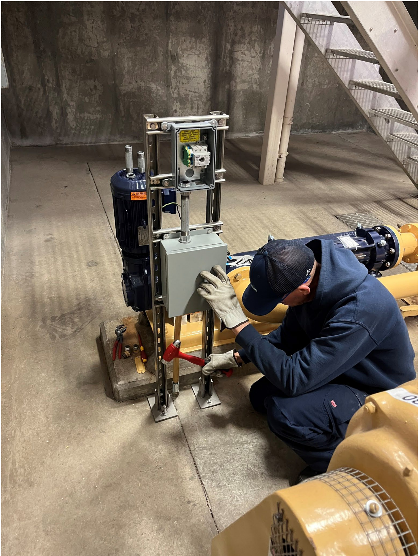
Primary Scum Pump Installation
