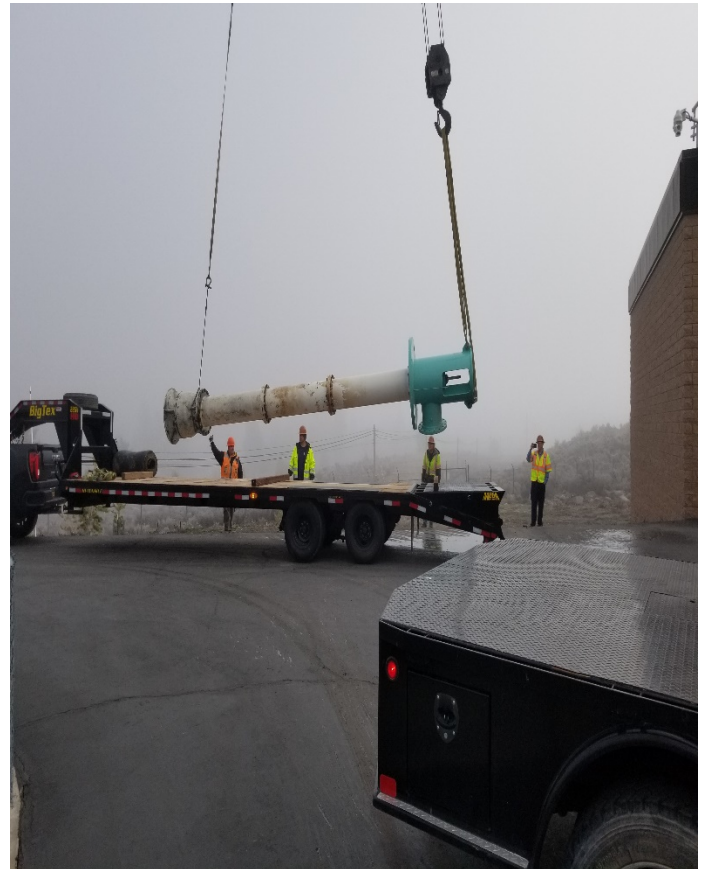
Loading of BNR influent pump #1
