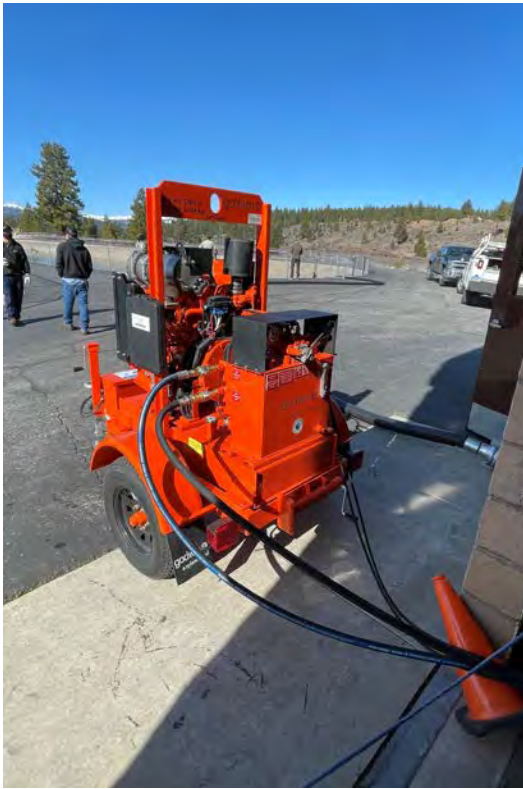
Submersible Pump and Power Pack Project Equipment Delivery & Testing
