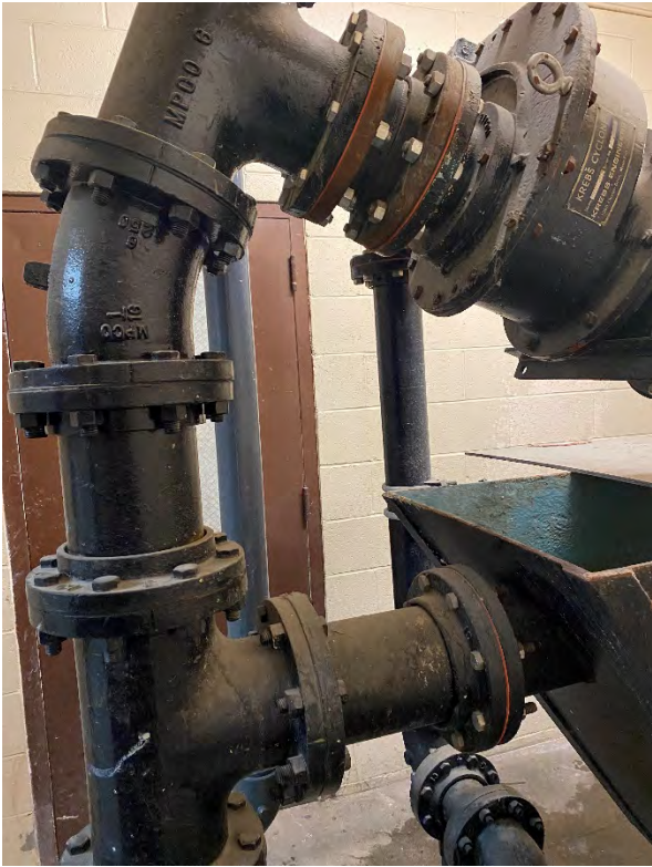
Out of Service Grit Classifier Removal
