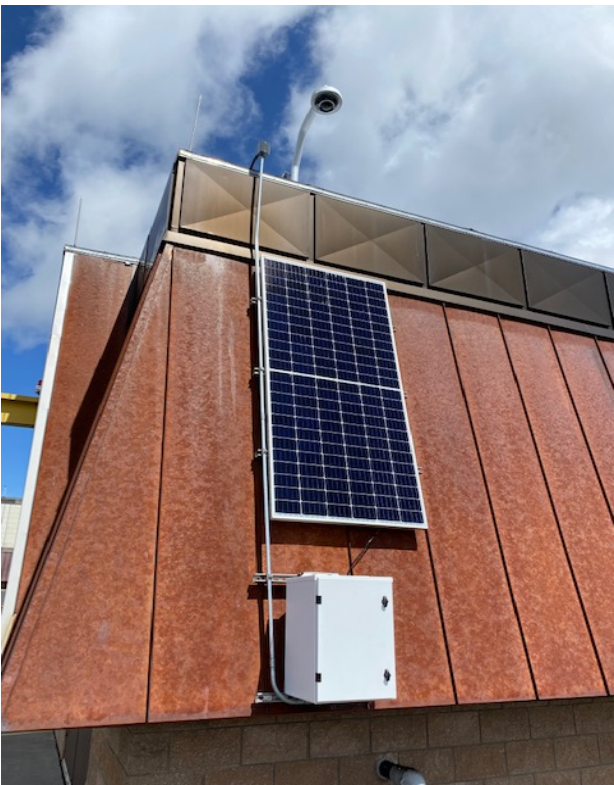
Solar powerd security camera chlorine building
