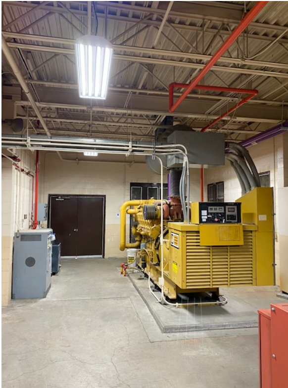
LED Lighting emergency generator room
