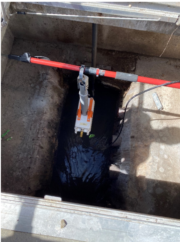
Flo-Dar meter installation
