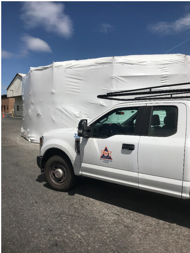
2020 Plant Painting Project – Relocated Floating Cover
