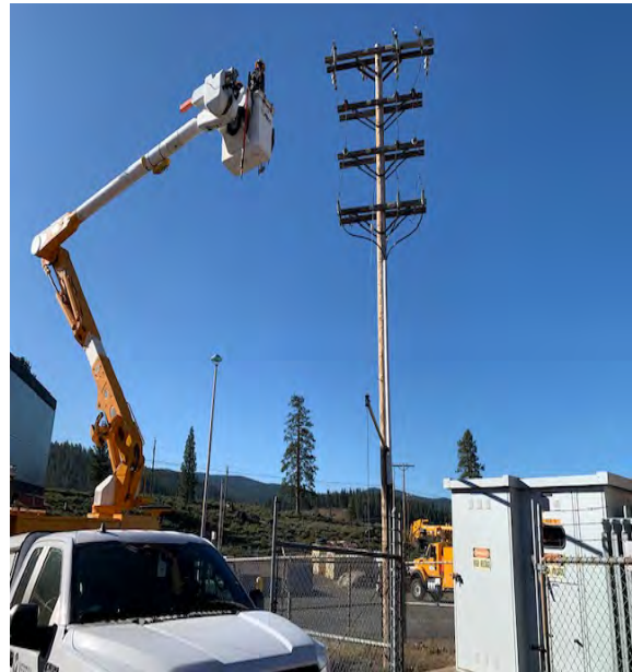
12 kV service (TUPD isolation of power)
