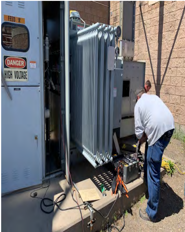
12kV power service
