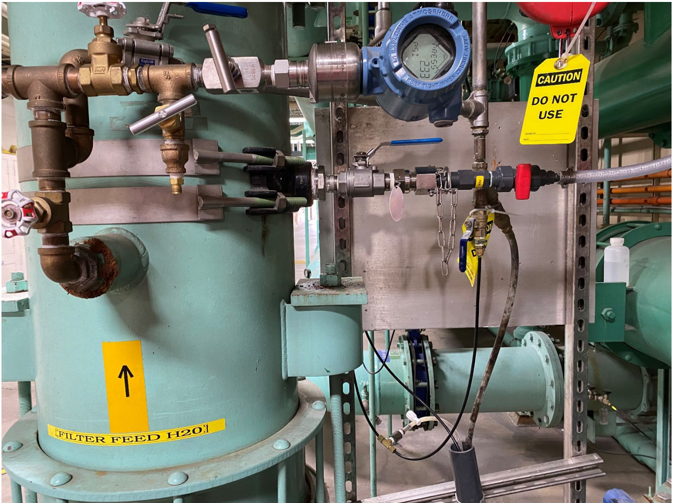
Filter Influent Chlorine Injection Quill
