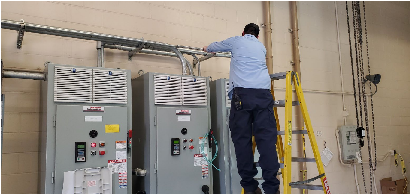
Profibus Communication Hub Installation
