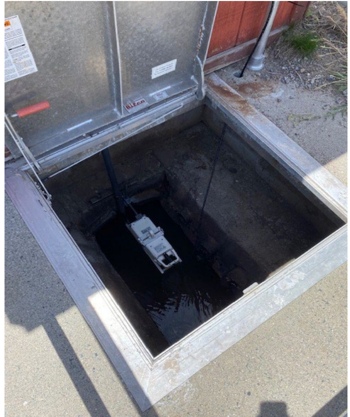
Flo-Dar flowmeter installation
