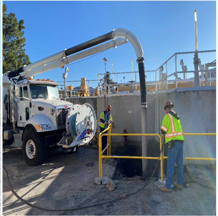
2 Water leak at O2 basin
