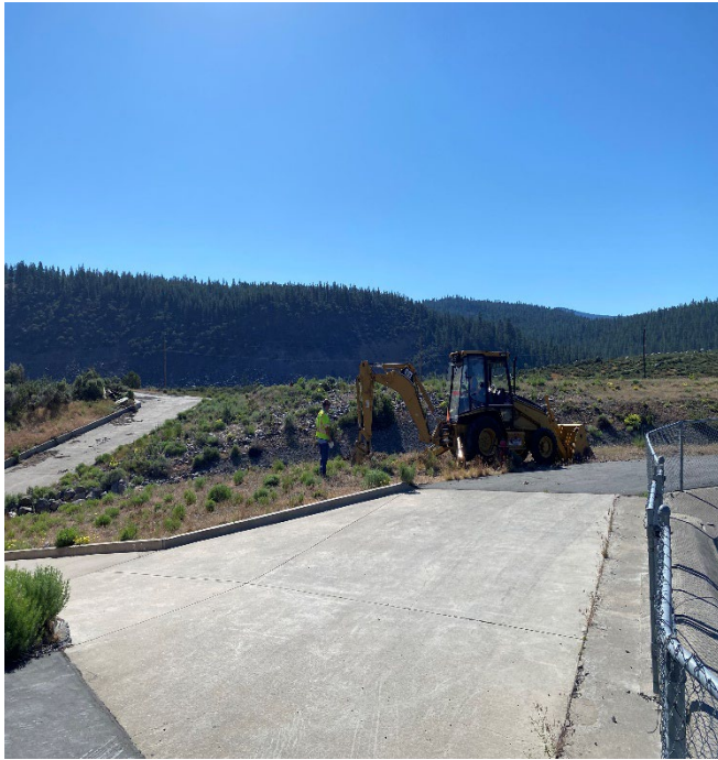
2 Water leak at ballast pond
