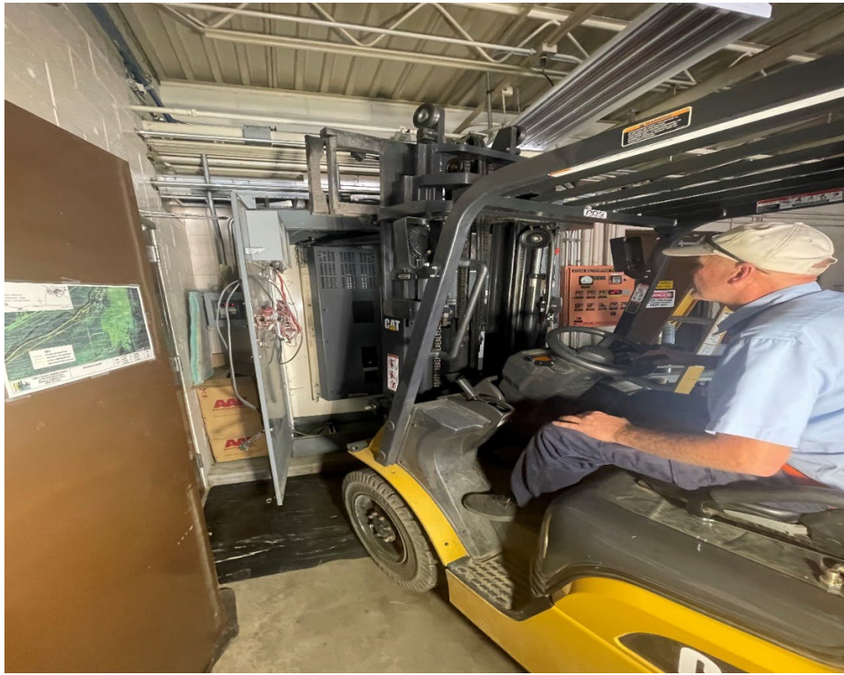
Multi-Purpose Pump Station VFD Upgrade
