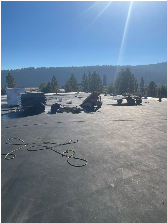
2023 Roof Repair Project Roof Removal and Staging on the upper AWT Roof
