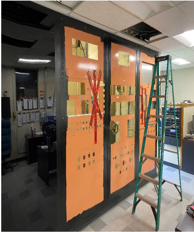
AWT Control Panel PLC Demo Work
