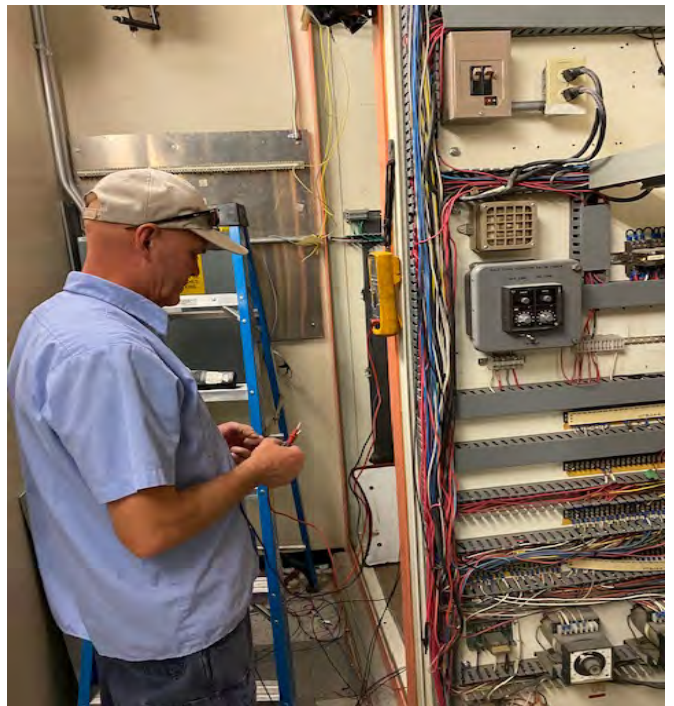
Chlorine Alarm Panel Upgrades
