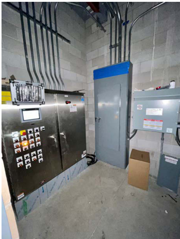
2020 Headworks Improvements Project New Electrical Room
