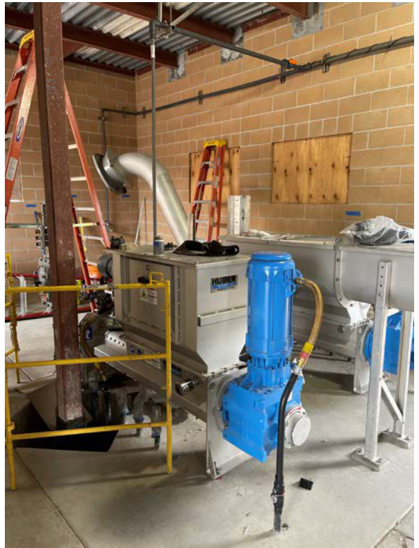
2020 Headworks Improvements Project New Screenings Wash Press
