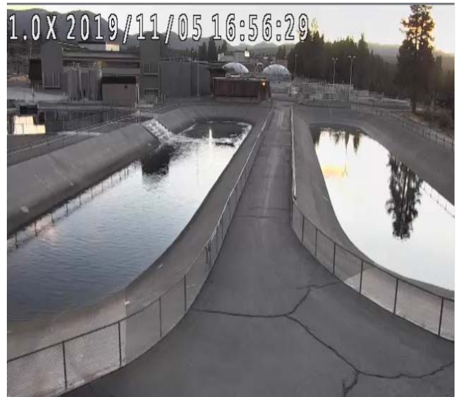
BNR Influent Pump Station Camera View
