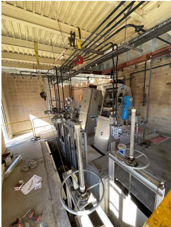
2020 Headworks Improvements Project Both Multi-Rake Bar Screens Installed
