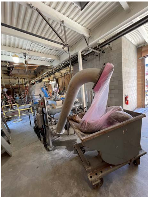
2020 Headworks Improvements Project New Screenings Wash-Press in Operation
