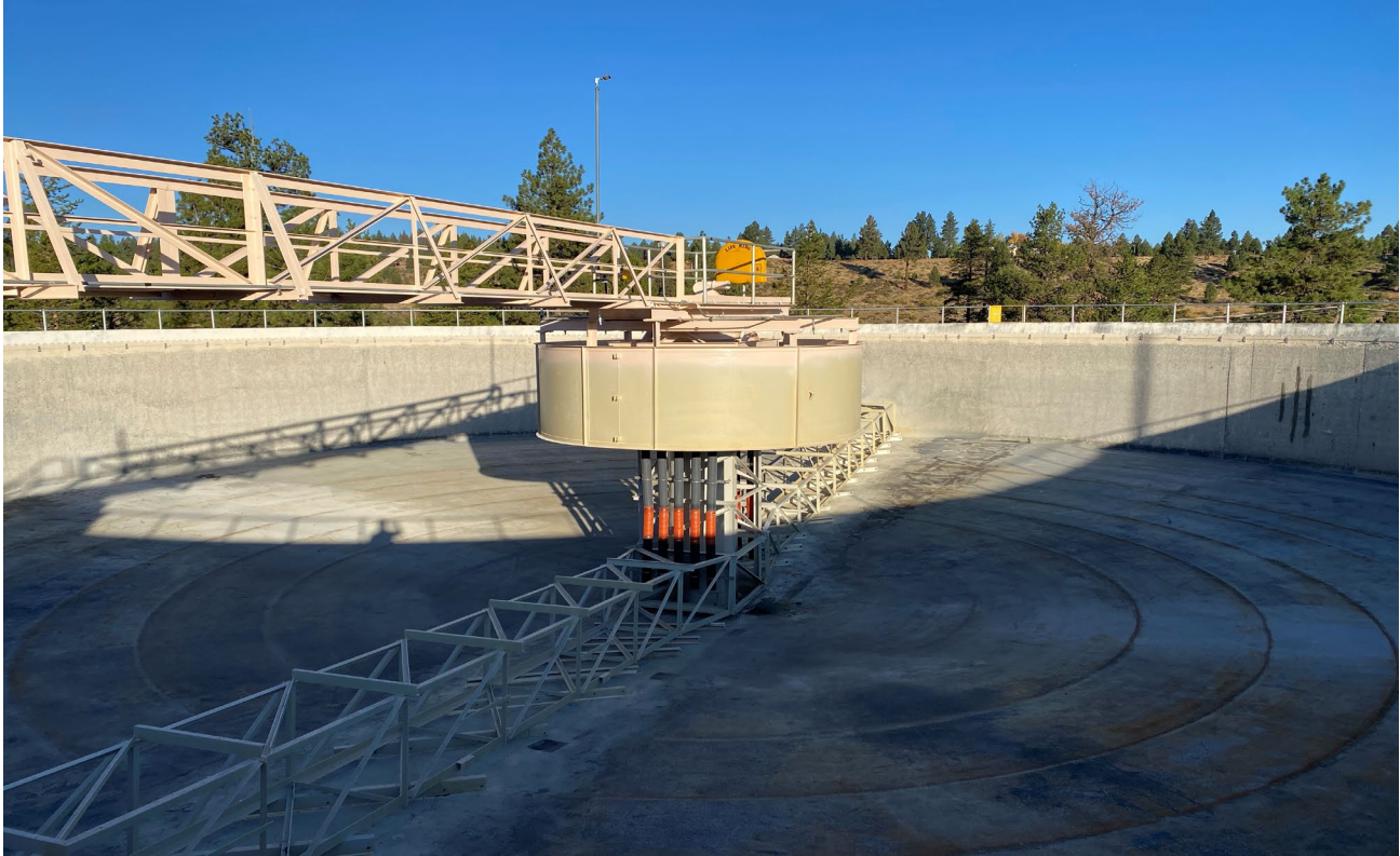
Clarifier Draft Tubes
