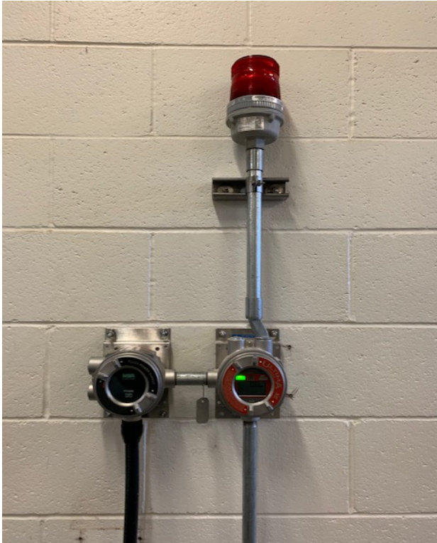
Chlorine Early Detection Alarm
