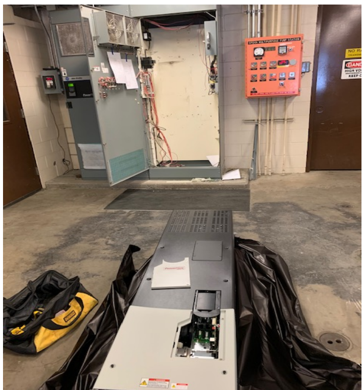
MPPS VFD Replacement
