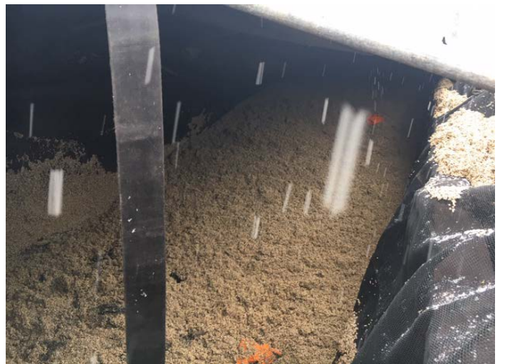
BNR Backwash Tank Bead Removal
