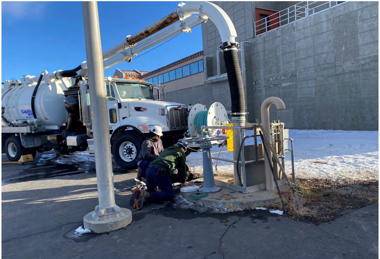
Plant Waste Pump/Wetwell
