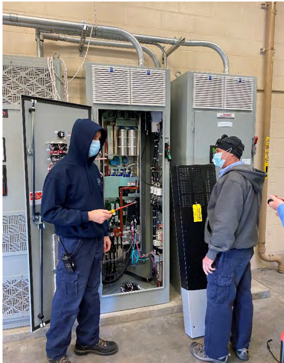
BNR Influent Pump VFD #2
