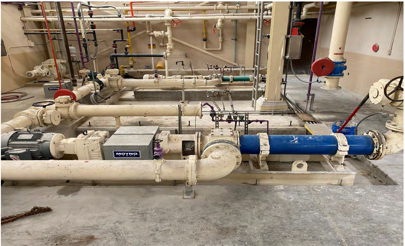
Moyno Filter Press Feed Pump Removal
