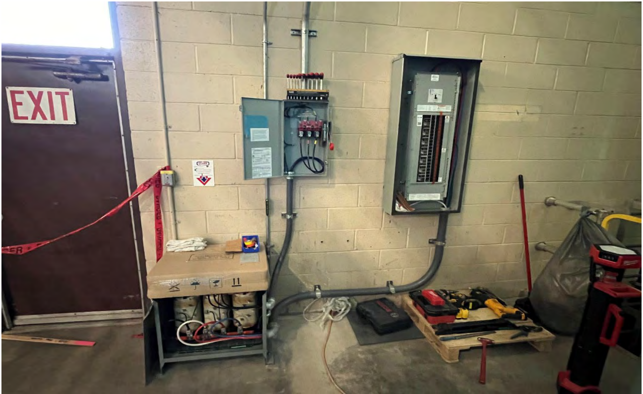
Sodium Hypochlorite Electrical Installation
