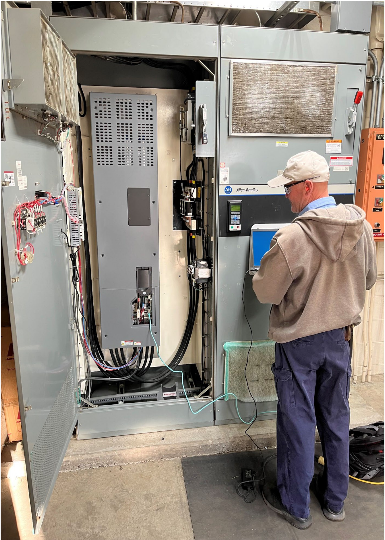
Multi-Purpose Pump Station VFD Configuration
