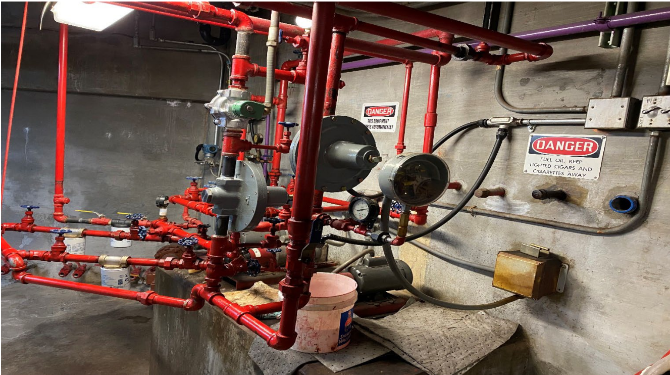
Fuel Oil System Regulators and Solenoids
