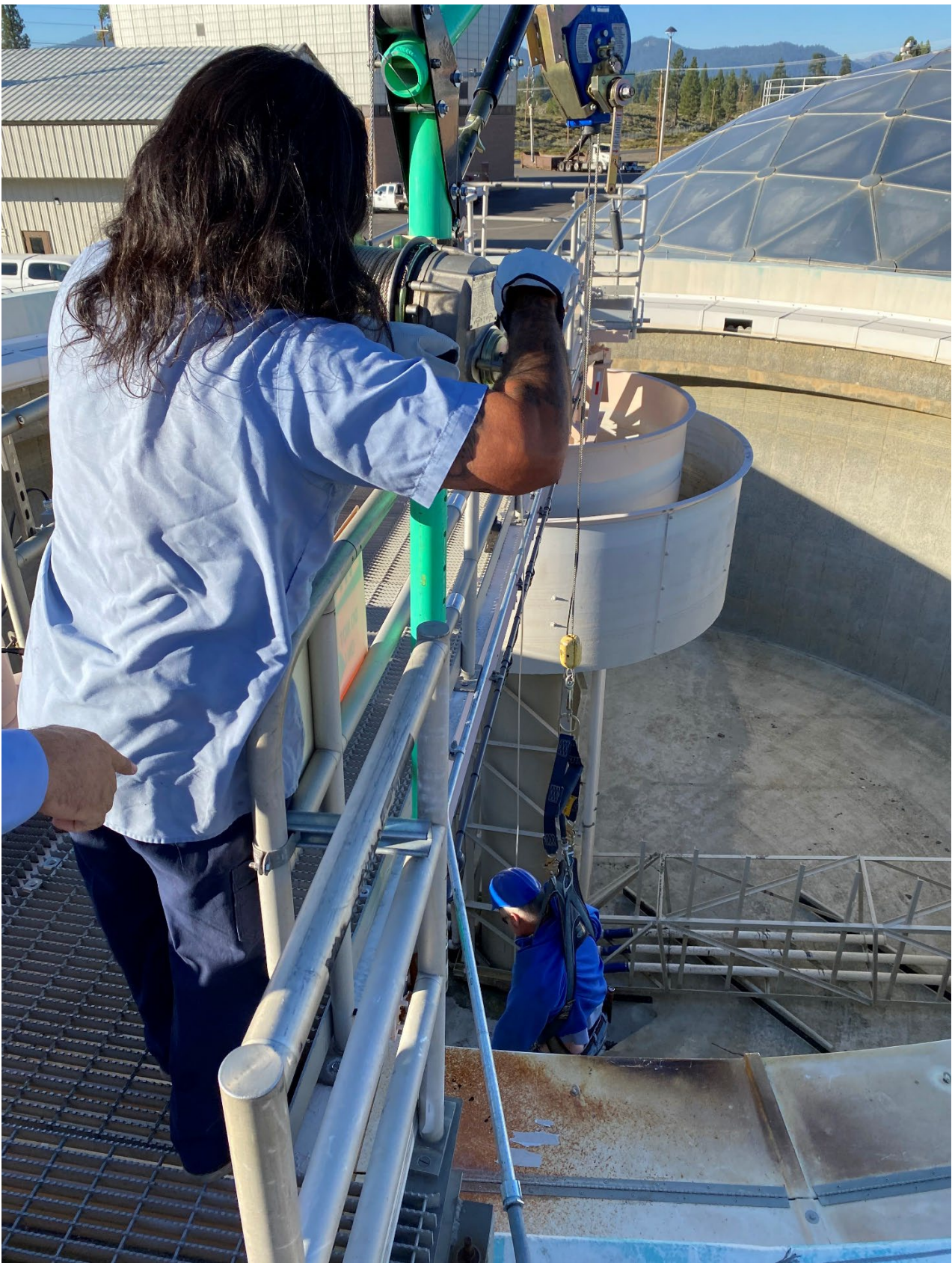
Phosphorus Stripper Inspection Retrieval
