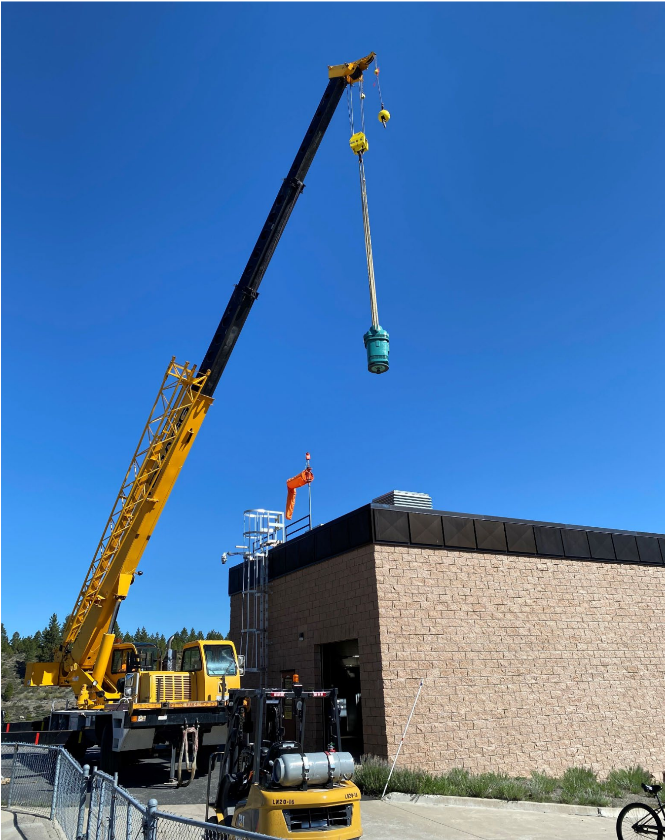
BNR Influent Pump Motor
