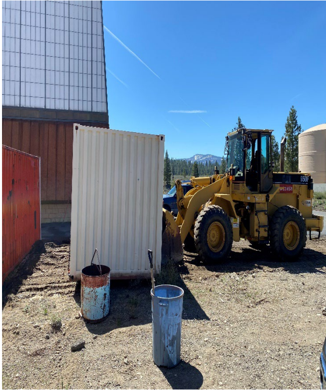
AWT Storage Containers
