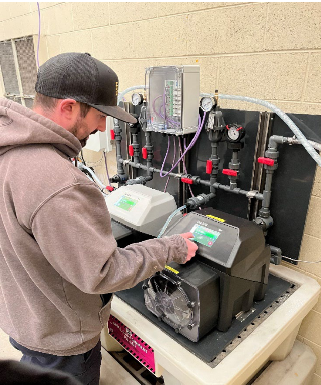
Sodium Hypochlorite Skid
